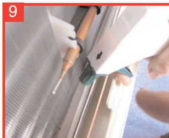
9 Clean the drain tray as required by spraying with AC-OK if accessible.
